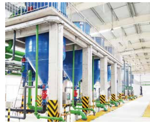
Membrane chemical reactor (MCR)
